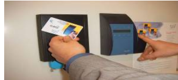
Building access control, security
